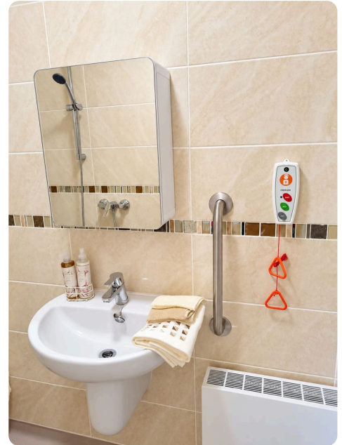
An en-suite, with a grab rail and an alarm pull-cord.
